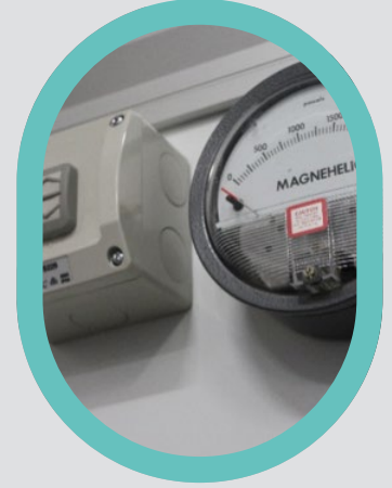
Magnehelic gauges and service lights
