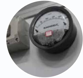
MAGNEHELIC GAUGES & SERVICE LIGHTS
