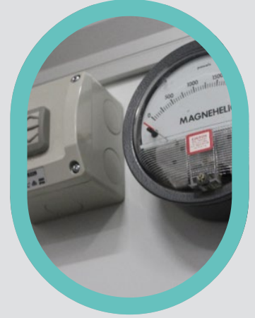
Magnehelic gauges and service lights
